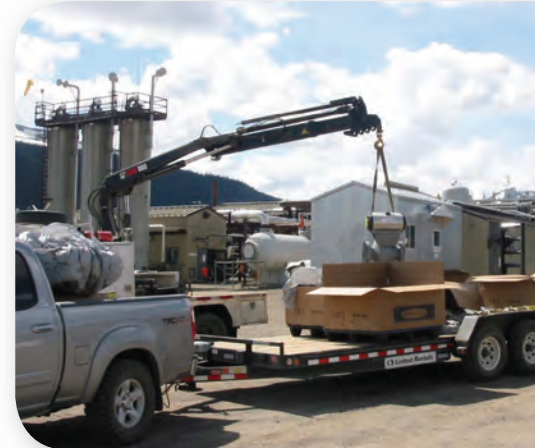
VTI valves arriving at gas plant.
