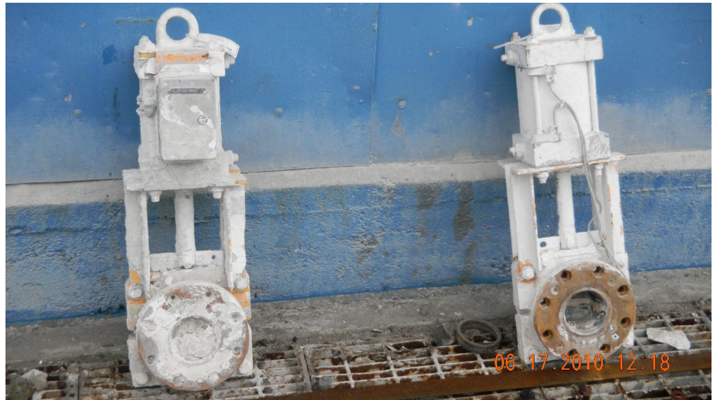
The Clarkson KGD valve used at the El Teniente plant
