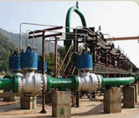
Figure 1: Station isolation valves – where the pipeline needs zero leakage to isolate long portions of piping & pressure reducing stations.
