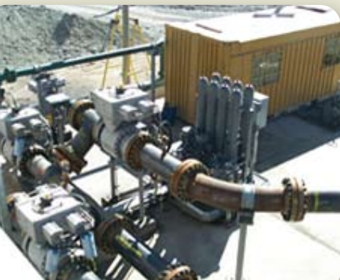
Figure 2: Main-line pump isolation valves – where zero leakage is required to isolate operating from non-operating pumps.
